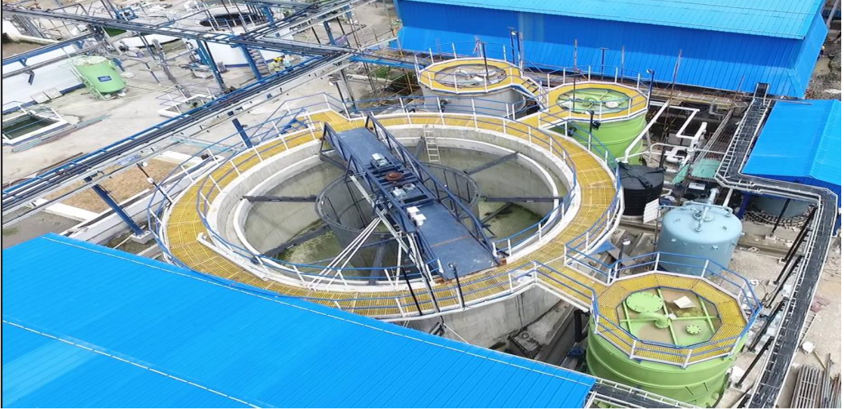
Effluent Recycling Plant Overview (40 m 3 /hr)
