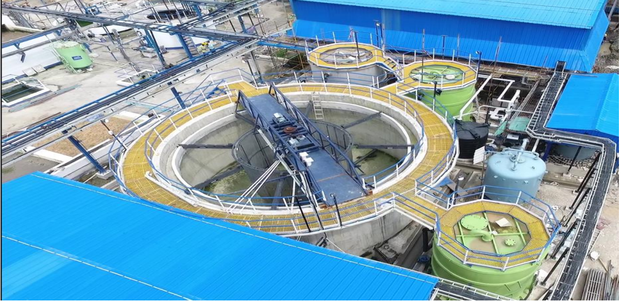
Effluent Recycling Plant Overview (40 m 3 /hr)
